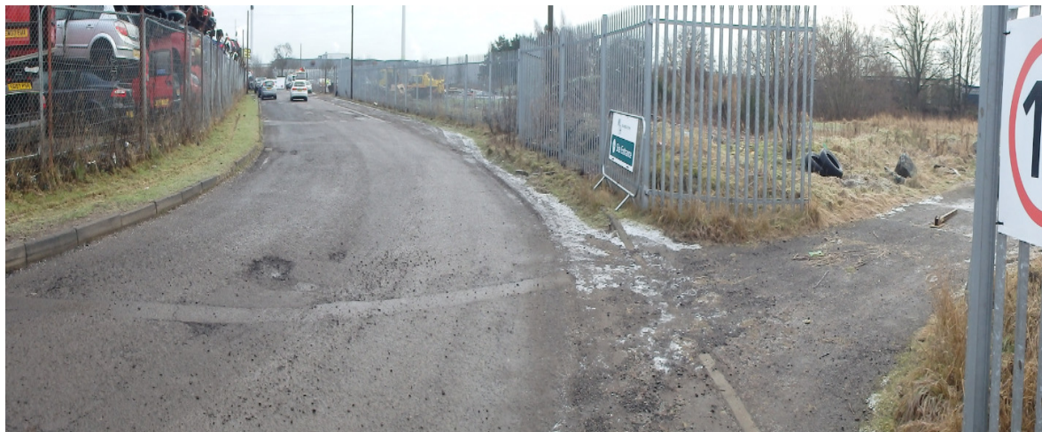
Figure 11b: Silt deposited on Beryl Street (Arup, 19/1/16)
