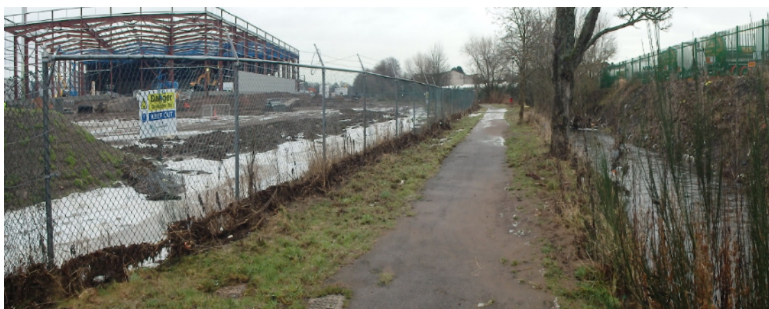
Figure 12a: Left bank footpath showing silt. Anecdotal evidence suggests flooding extending into to the manhole located within the fenced area. Location 6, Figure 5. (Arup, 19/12/16).
