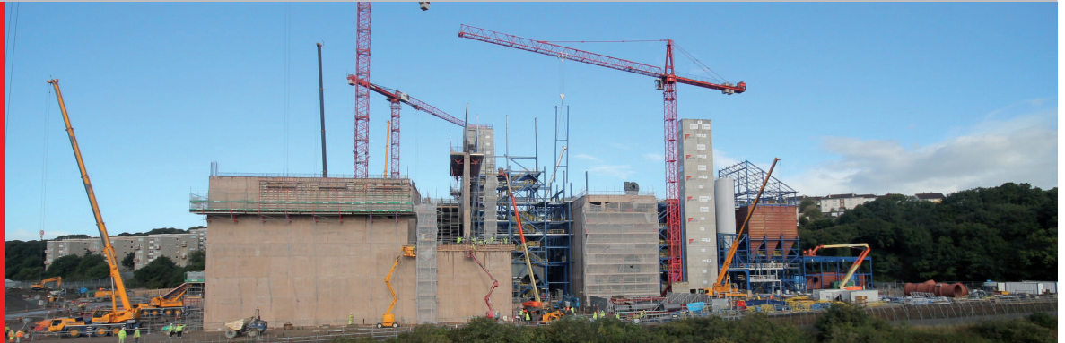
This recent picture from our webcam shows (from left to right) the waste bunker wall, followed by the boiler house, the turbine hall and the APC residue containers. The chimney will be erected at the far right of the picture.
