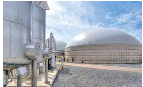
The biomethane plant at Stassfurt in the Magdeburger Börde region
