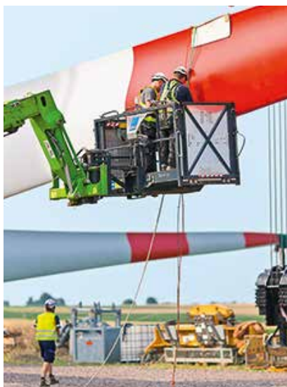
Working on the rotor blade at a wind turbine in Offenbach an der Queich
