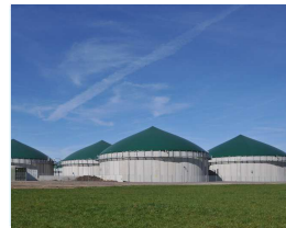
Further developing our biomethane activities
