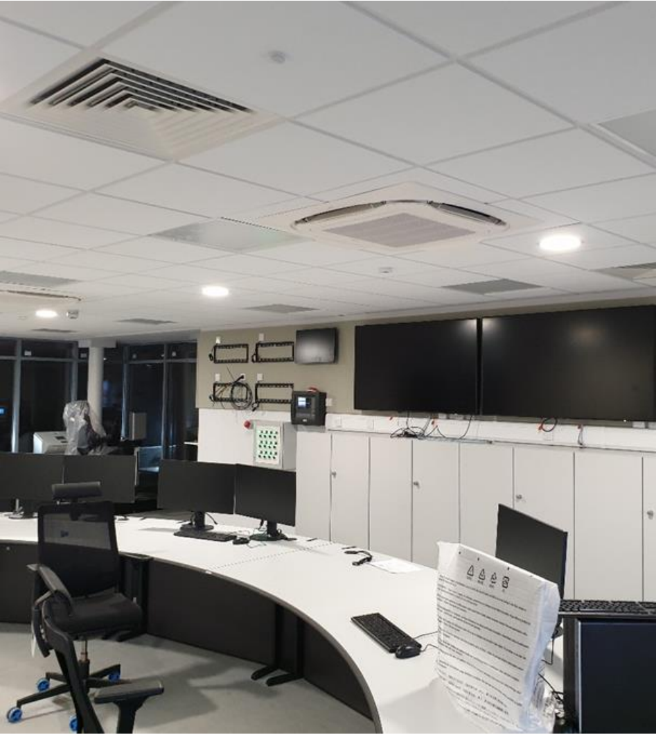
Control Room furnished and Monitors installed
